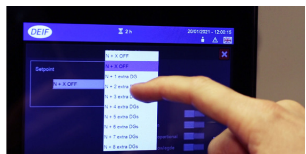
The new N+X feature. You decide how many extra gensets should be running in a given load situation
